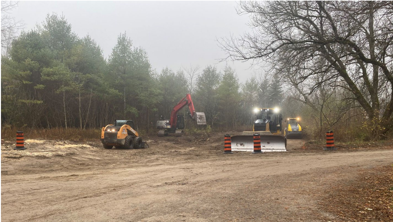
Photo 1: Removing woody material and topsoil from expansion area and starting proof roll of base
