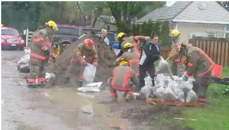
Fire crews and residents spent Thursday filling sandbags and creating a blockade around dozens of waterfront houses in Bowmanville's Cedar Crest Beach community. (CTV News Toronto)
